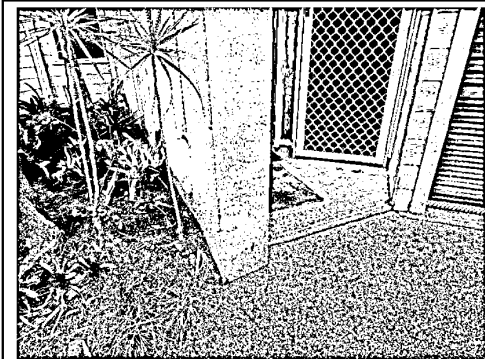
High soil, paths and gardens about the external walls. This could provide hidden access to termites.
