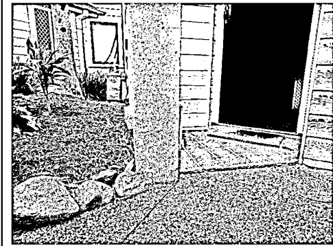
Unit 2. High soil, paths and gardens abut the external walls. This could provide hidden access to termites.
